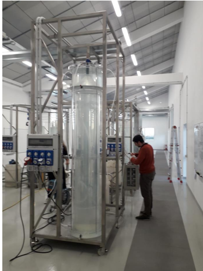
Figure 3. Power to gas plant installed
